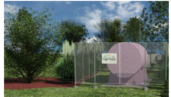
Water surge control vessels at Horton Park
